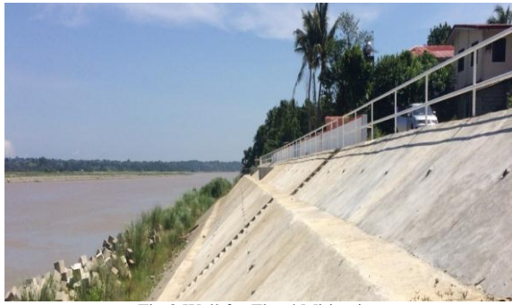
Fig.2 Wall for Flood Mitigation
